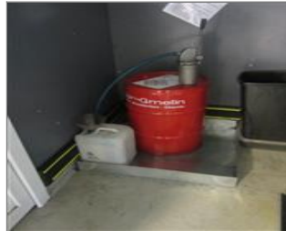
Photo of the inside of the main production hall Secondary Containment.JPG
